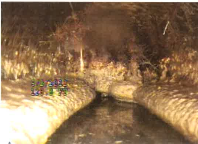
Figure 1: Buildup of grease causes a decrease in pipe diameter, courtesy; City of Dover
