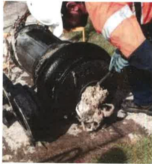
Figure 4: Materials clogging a pump station ( www.theage.com.au )
