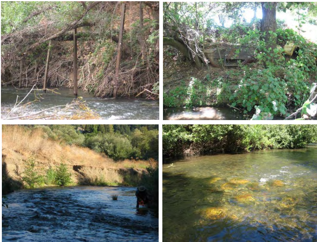
Figure 34: (upper left) Failed I-beam and chainlink fence stabilization efforts, (upper right) car bodies in the banks, (lower left) erosion along an outside bend, (lower right) a triangular boulder cluster in Dry Creek.
