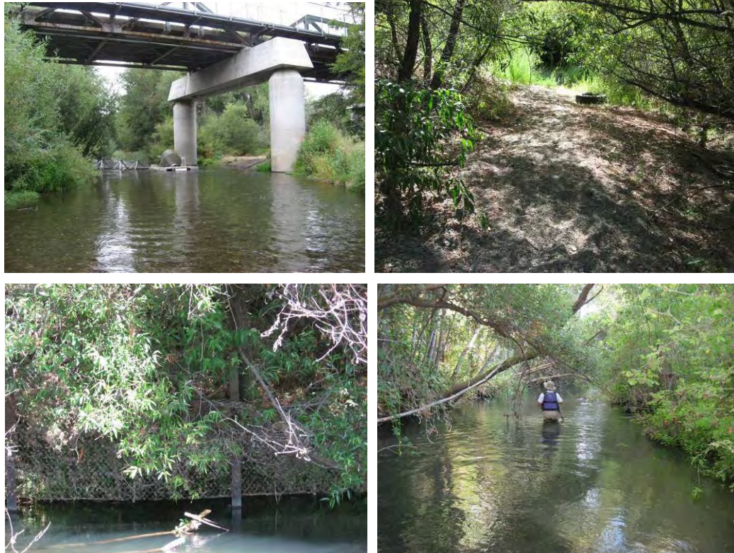
Figure 12: (upper left) Westside Road bridge and screw trap, (upper right) mouth of intermittent stream, (lower left) failed I-beam and chainlink bank armor, and (lower right) side channel pool.
