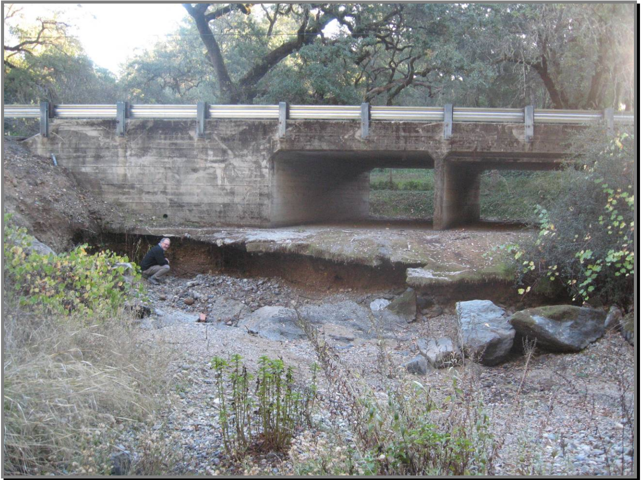
Photograph 4: Evidence of stream bed incision in Dutcher Creek, below the Dutcher Creek Road Bridge.
