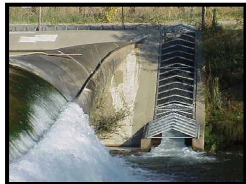
Inflatable dam (left) and fish ladder (right)
