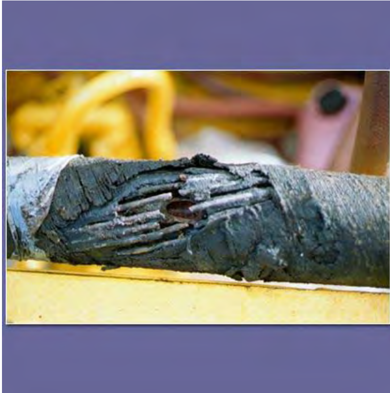
Figure 3-1 Physical Damage to a 15 kV EPR Submarine Cable caused by a 1550-Ampere Fault (as it appeared coming aboard the Repair Barge)
