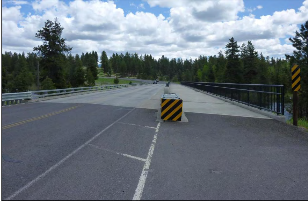
Figure 6 – Existing pathway over Deinhard Bridge (pathway on right, travel lane on left)
