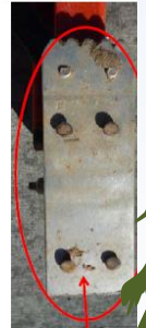
Missing Rubber cap
